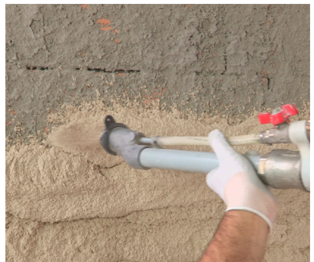
Application of an aerogel render with hydraulic lime as the main binder.
