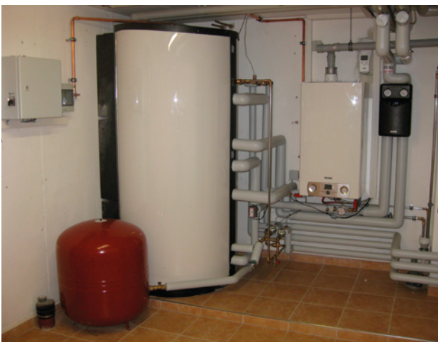
A 1 kW (electricity) \mu CHP system including thermal storage.
