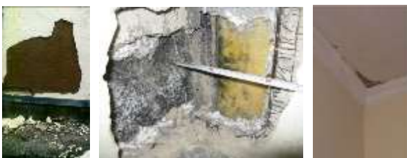
Figure 2.1 Identified failures due to inside insulation: Frost damage (Hartwig M. Künzle IBP 2011), left; Mould growth inside the exterior wall construction (Th. Bednar, TU Wien, 2012), middle; Mould growth at the junction of an inside insulated outer walls (S. Korjenic, TU Wien, 2007), right.
