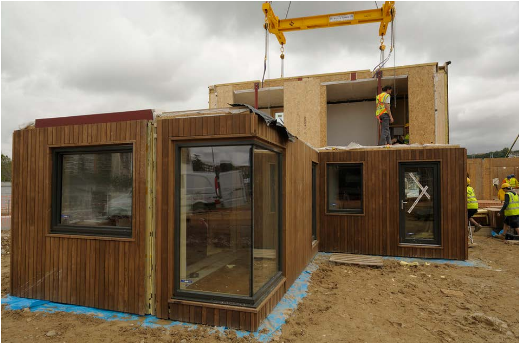
Figure 4-18: The Nottingham H.O.U.S.E being assembled. The four lower modules have already been assembled, the first upper module is currently being placed by crane. Source: Solar Decathlon Europe (SDE flickr, 2010)
