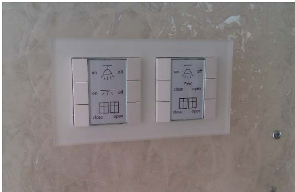
Figure 12-1: Typical low-voltage pushbuttons as part of the building automation system to replace classical switches for AC wiring (SDE 2012). Source: University of Wuppertal
