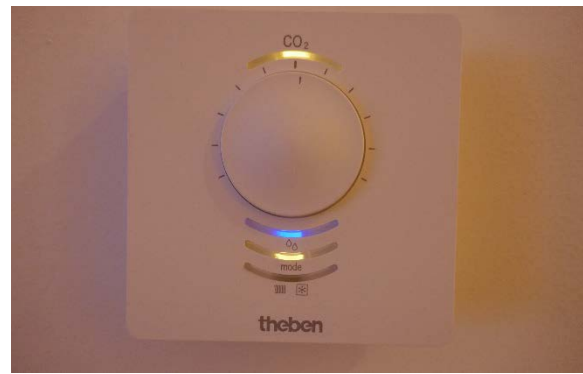
Figure 12-2: Turning knob to manually adjust the set point for a CO2-controlled ventilation system (SDME 2018). Source: University of Wuppertal
