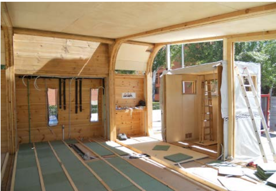
Figure 4-25: Interior view of the building during on-site construction. You can see that essentially only the wooden elements were delivered in the shell state. Source: Universidad Valladolid, Construction Drawings, page 9
