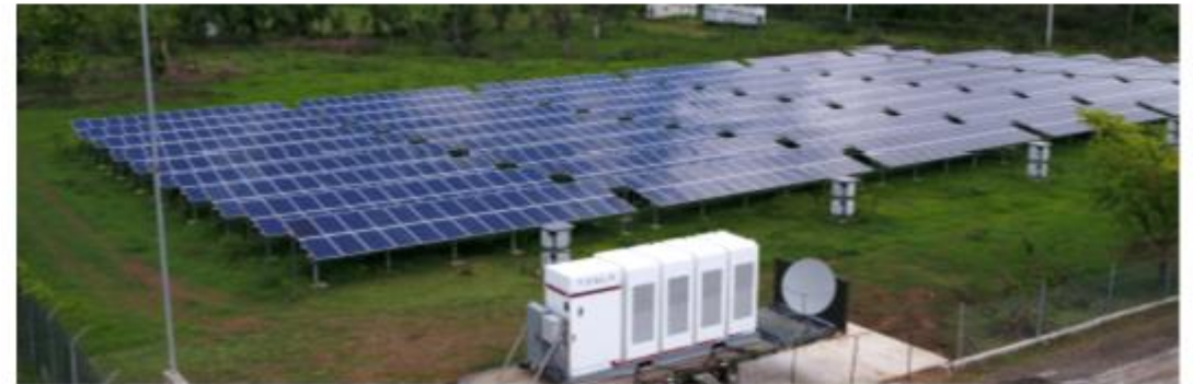
Figure 8.9. Emergency power generation using a PV panel field connected to a battery pack.
