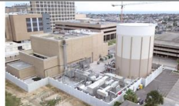
Figure 8.5e Equipment at a power plant is protected by a flood wall ((The University of Texas Medical Branch at Galveston)
