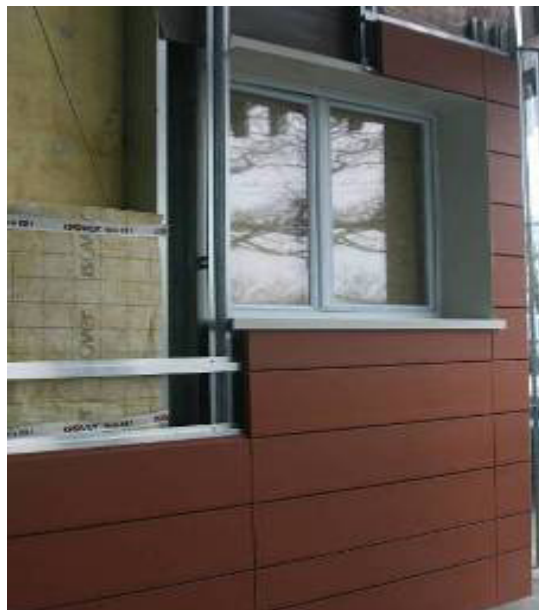
Figure 5. Metal supporting structure for the French multi-storey façade module (left); test installation (right).
