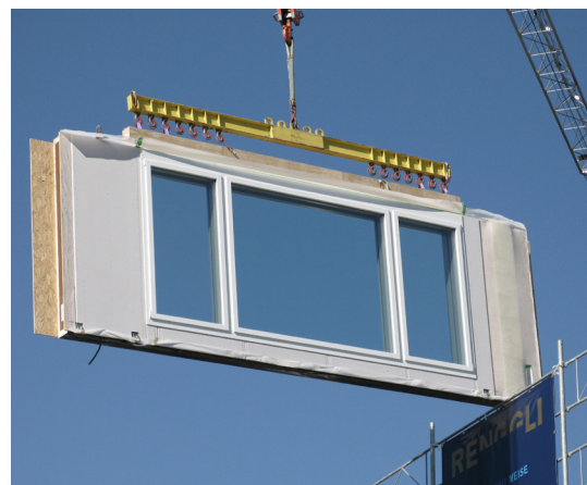
Figure 1. Prefabricated façade modules used to construct a new building envelope outside the existing building.
