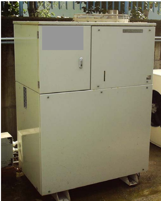
Fig. 13. Cogenerator considered in the case study.
