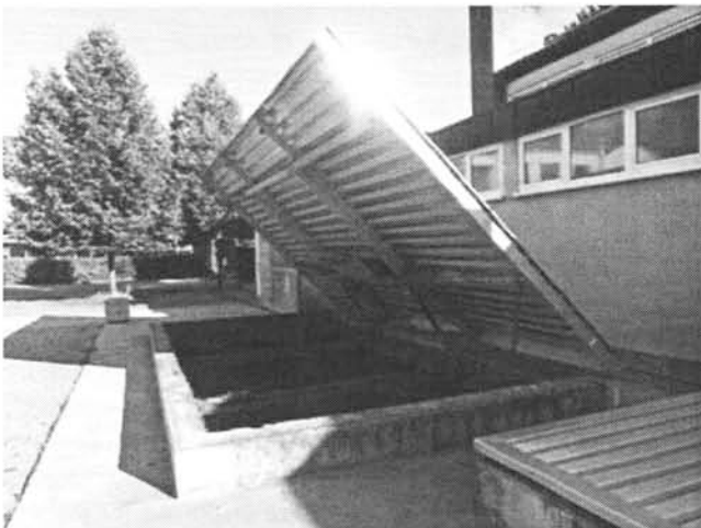
Figure 3 Wood-chip bunker on the school campus.
